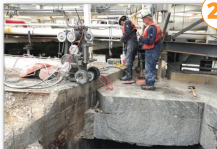
A crew from Advanced Coring & Cutting Corp. at work at the Kinder Morgan, Inc. storage facility in Perth Amboy, NJ.
