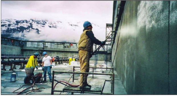
A protective layer of crystalline waterproofing is applied to the Valdez Marine Terminal water purifying tanks in Prince William Sound, Alaska.
